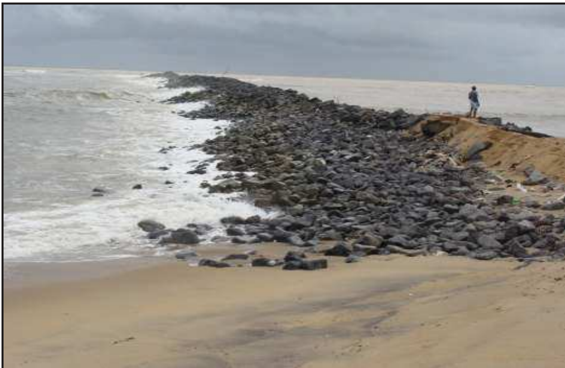
Figure 10: Ullal Breakwater during 2010. The Breakwater Severely Damaged.
